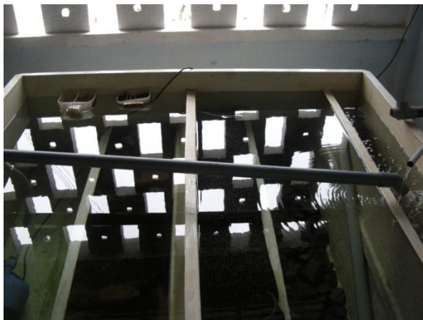
Figure 23: This is one of the many filters on the facility.
